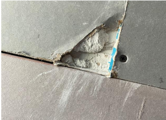
Figure 14-2. Sheetrock Broken Corner.
