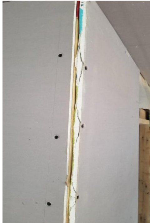
Figure 14-5. Cracking Resulting From One Proud Corner Stud.
