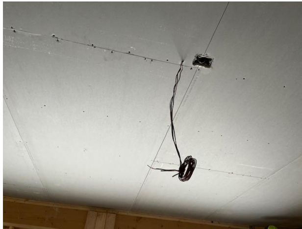
Figure 13-5. Exposing Garage Door Opener Wire.
