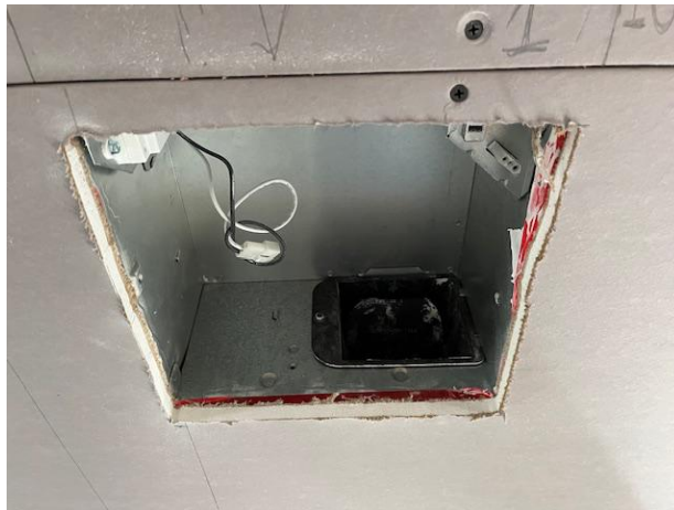
Figure 13-4. Damaged Tape Seal from Spiral Saw Cut-Out for Bath Fan.
