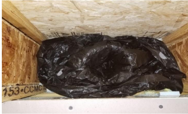
Figure 12-1. Plastic Bag Inserted Into Future Fan Vent Duct.
