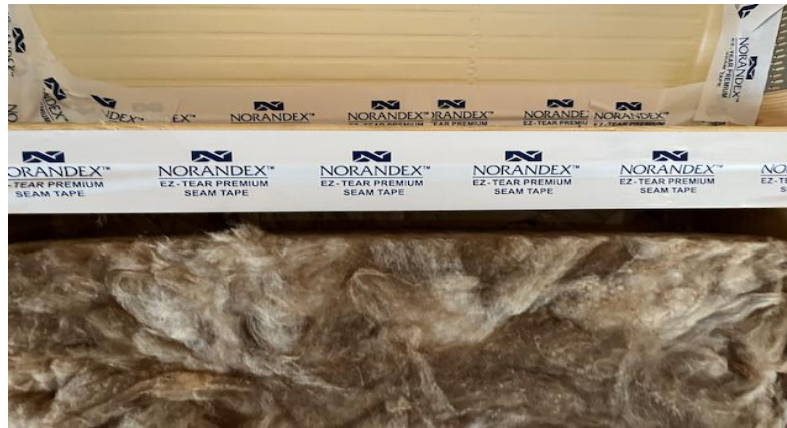
Figure 12-6. Air Gap Between Insulation and Upper Plate.
