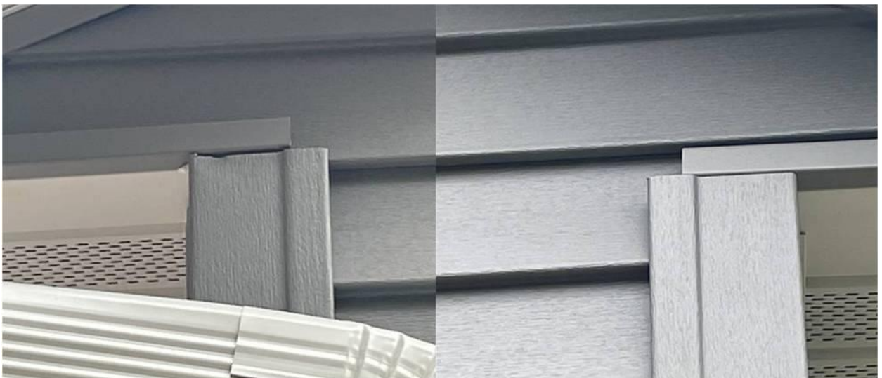
Figure 11-9. Unacceptable J-channel Installation.
