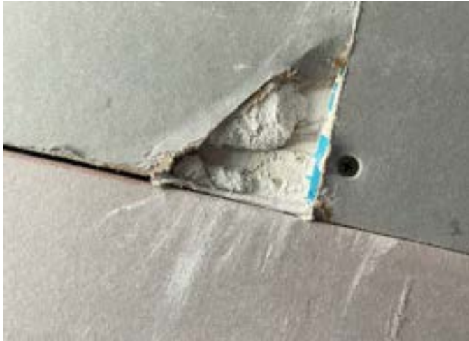
Figure 14-2. Sheetrock Broken Corner.
